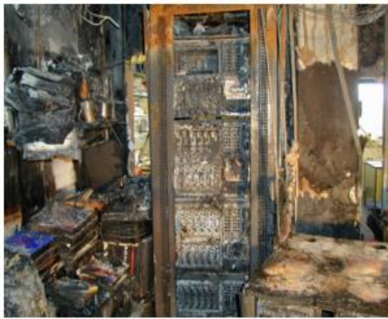
Fire Destroys Data Center
